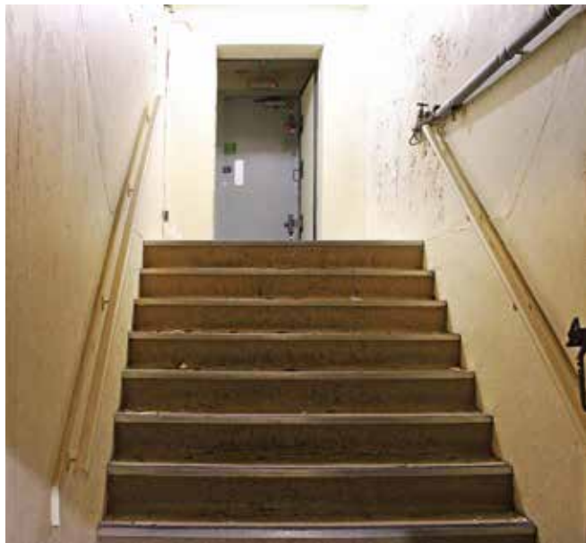
Interior view of access stairs looking towards main blast door at surface level. Stairs were constructed as part of the 1980's bunker alterations
